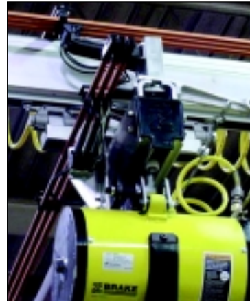
Electric supply using Insul-8
